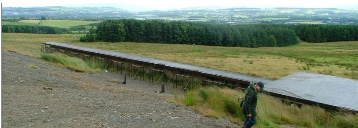
The combined erosive forces of running water and gravity try hard to bury the gallery under a slow, but steady landslide.
